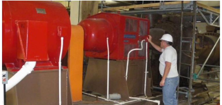
Photo courtesy Lemay Pump Station
