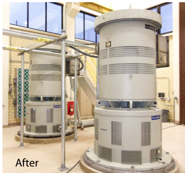
Top: Ideal Electric Units CAV61320 vintage 1976 unit Above: Dynamatic SPMV-8260 unit Both installations are rated 1250hp, 514rpm, 4160 volts
